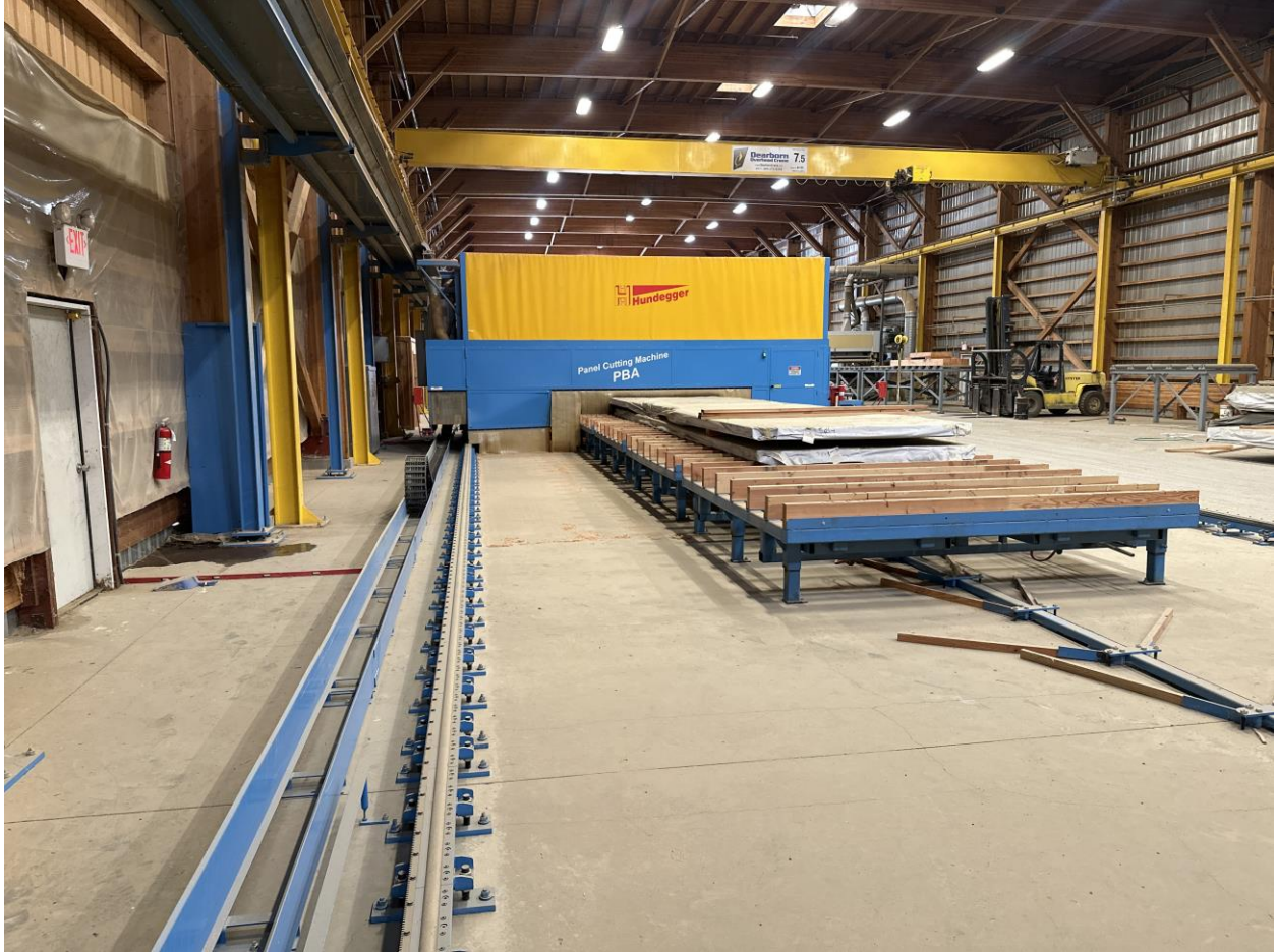
The powered roller system was installed, but never commissioned.
