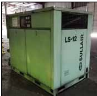
SULLAIR LS-12 60-HP Air Compressor
