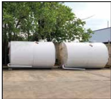
(3) 4,200-Gallon Storage Tanks
