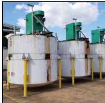
(4) TSM 2,500-Gallon Let Down Tanks w/SCHOLD Agitators
