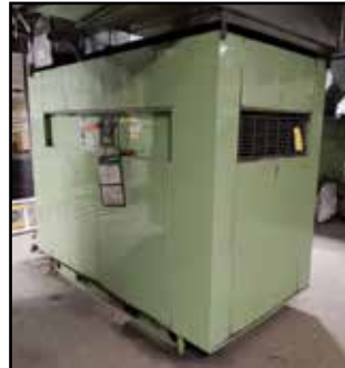
(2) SULLAIR LS-20 100-HP Air Compressors
