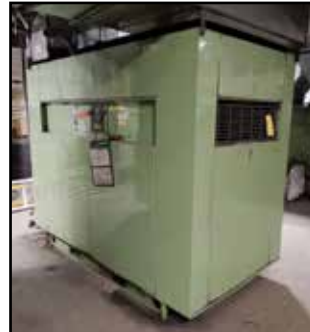
(2) SULLAIR LS-20 100-HP Air Compressors
